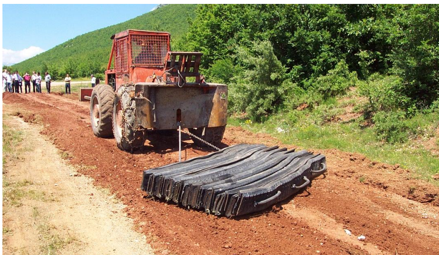
Forest road maintenance is an important part of the forest supply chain. Here the rubber grader is being pulled by a skidder.
