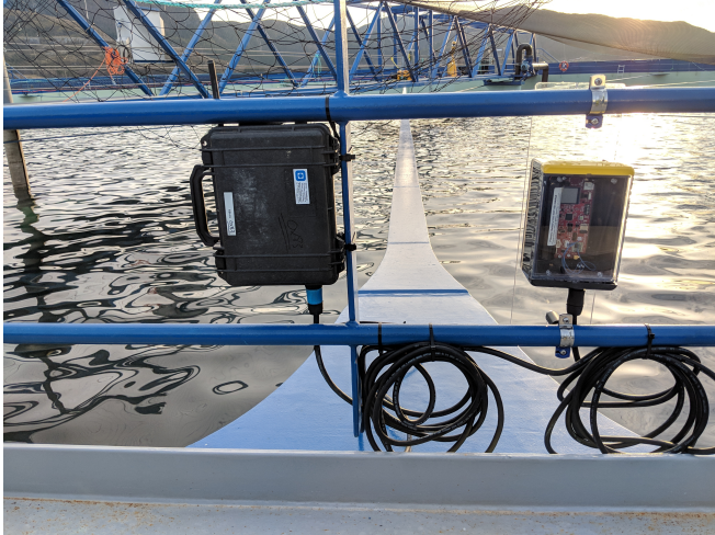
Fig. 4 SLIM nodes installed in redundant configuration on cage structure
